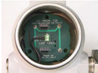
Photograph No. 2 Termination Board
